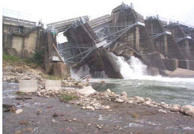
Fig. 7 Shear failure of Shigang dam
