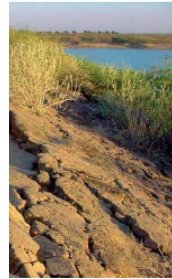
ge of embankment dams caused ularat province, India, January and water supply were damaged. ings on top of intake towers of the n earthquake
