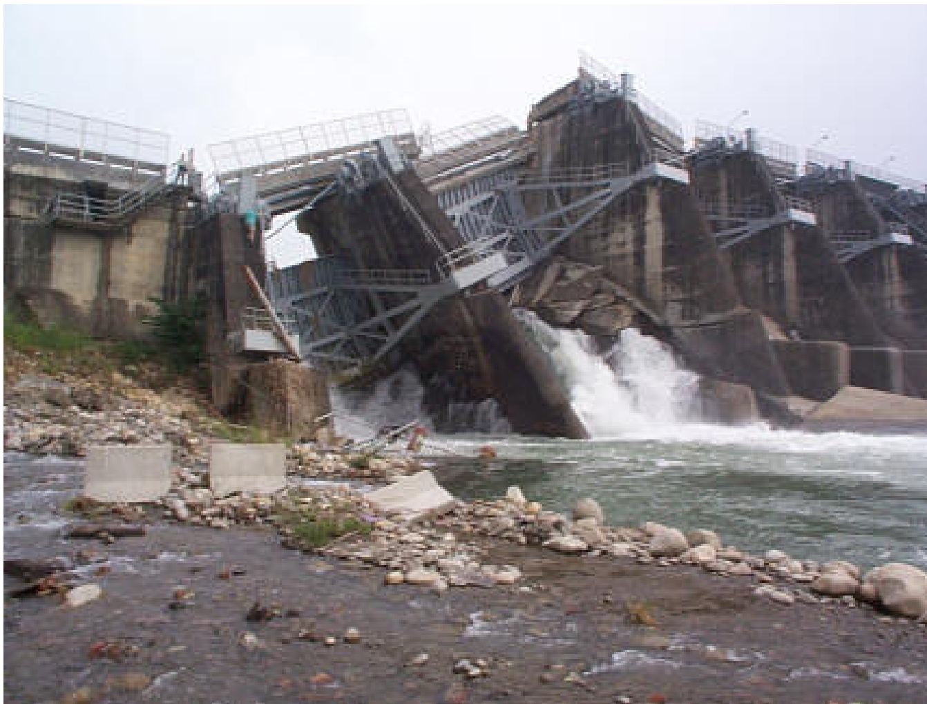
Shear failure of Shigang dam
