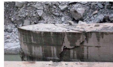
case of the Wenchuan earthquake, a large number of rockfalls took place, which caused signi- cant damage to dams and appurtenant structures. Surface powerhouses were particularly vulnerable to rockfalls in the steep valleys in the epicentral region of the Wenchuan earthquake.
